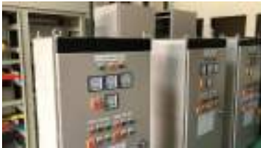
Sub Distribution Panel
