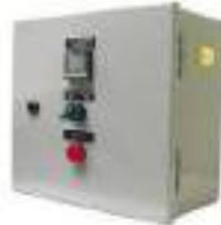
Temperatur Control Panel
